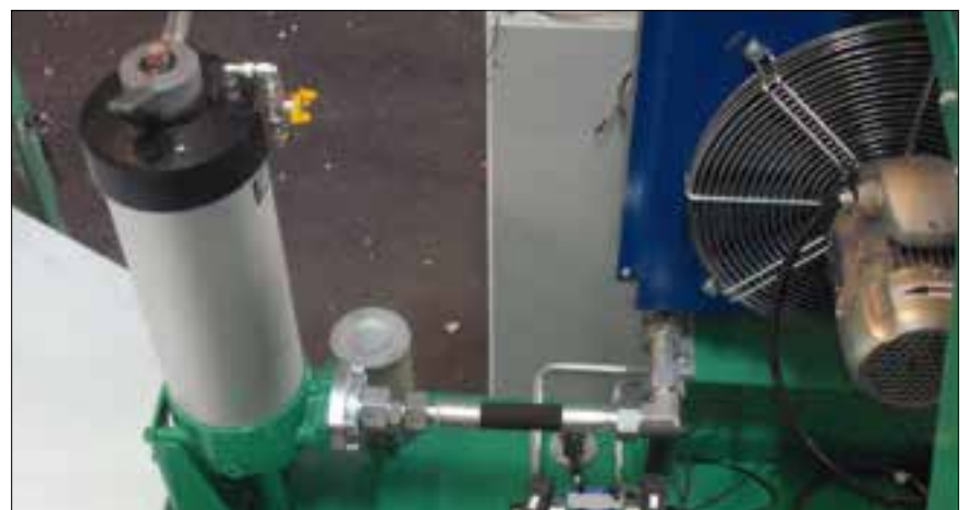
Figure 10. Offline circuit for filtration and cooling
