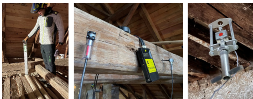
Figure 1: Illustration of the methods utilised to assess the structural health of wooden construction in the castle: resistograph, Measurement of the transit time and screw withdrawal.
