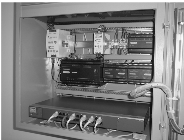
Figure 7: View of an experimental setup with RTU devices for microgrid experimentations.
