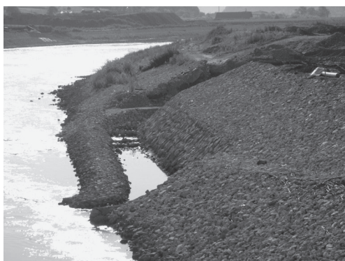
Slika 3: HE Blanca - vhod v obtočni kanal Fig. 3: Blanca HPP - entrance to the bypass channel
