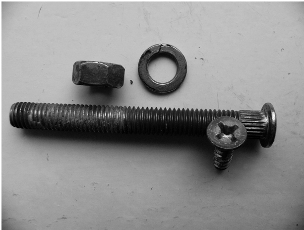
Figure 3: A nut, a spring washer, a structural bolt of the stairs and a cross-head screw, all covered with rust
