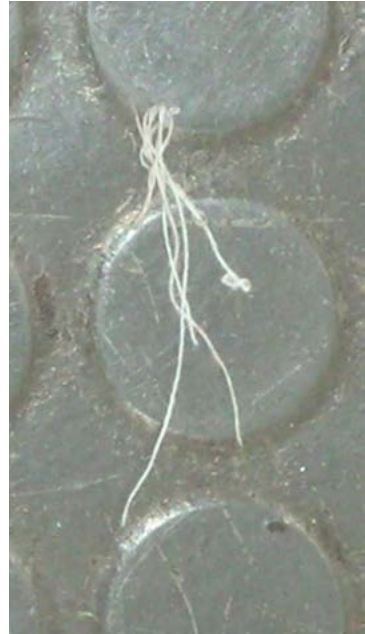
Figure 1: Scratch on the floor. Photo: MB.
