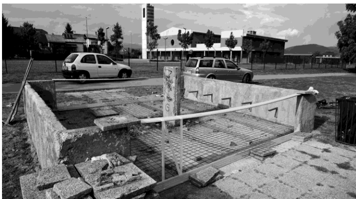
Figure 4: Action planning – renovation of the water well on the playground in Zalog as part of urban acupuncture process (photo: Domen Grögl).
