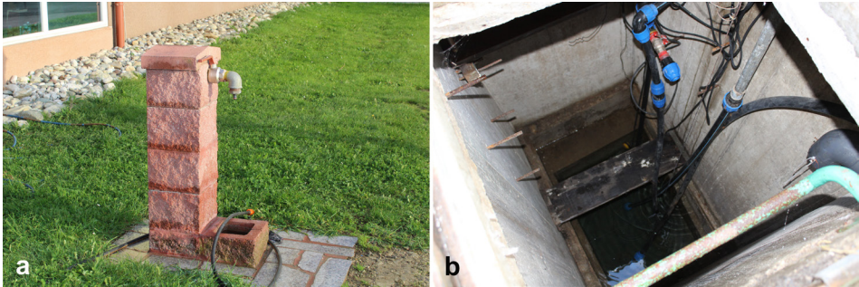
Figure 4: Example of a borehole (a – sampling site – borehole P6) and a well (b – sampling site – well P9) at selected sites.
