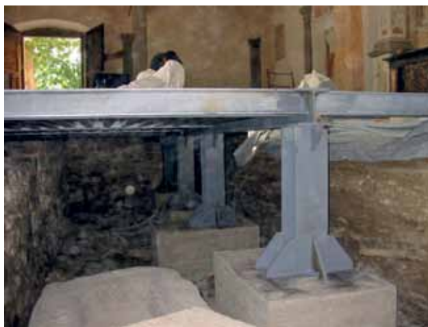
Fig. 17: Santa Maria del Lavello, the foundation of the pillars in the opaque part of the pavement (Courtesy of G. Suardi).
