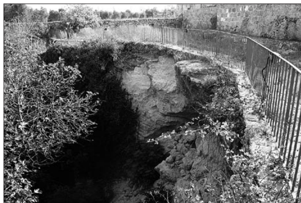
Fig. 5: Recent fall at the eastern margin of Vora Grande in February 2011 (Photo: M. Parise).
