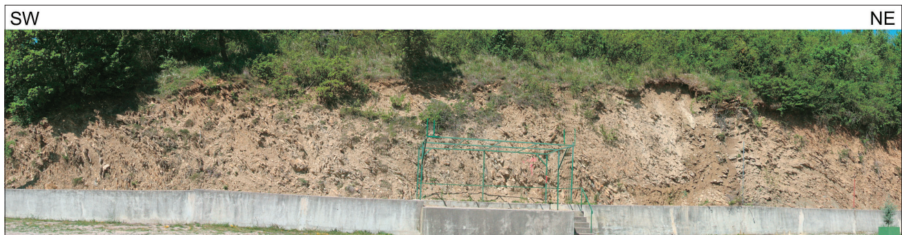
Fig. 13. Hrastovlje Thrust Fault , transversal section of part of the fault zone. Cut face behind hunter cabin in Kortine settlement. Fault zone in sandstones and siltstones. View from southeast to northwest.
