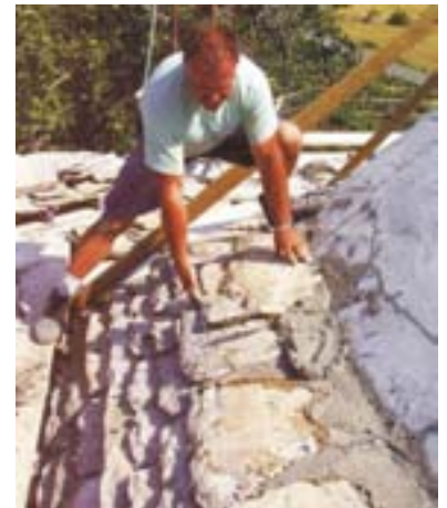
Slika 5: Polaganje skrl v malto pri obnovi cerkvene strehe v Križu pri Sežani. Laying slates in grout during renewal of the church roof in Križ, Sežana.
