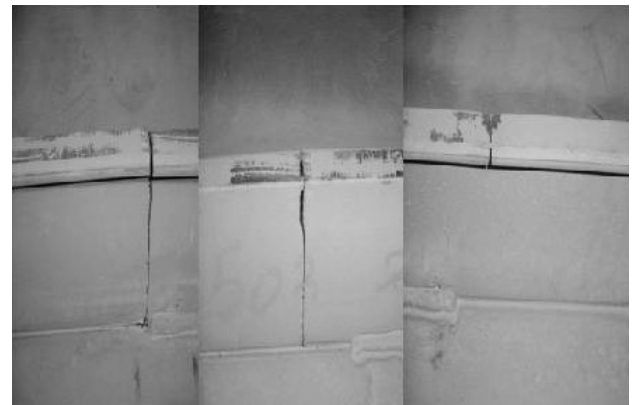
Figure 7: Cracks in the central stiffener, both sides and the lateral stiffener (after panel dismantling) Slika 7: Razpok v centralnem rebri, obe strani in bočna utrditev (po demontaži panela)
