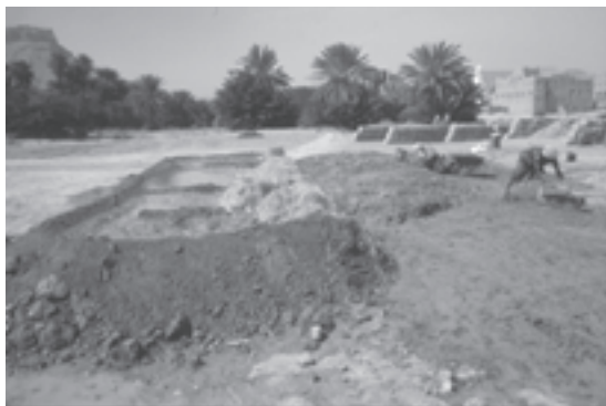
Slika 1: Ilovica po izkopu gradbene jame. (Foto: B. Juvanec) Clay after extraction from a clay pit.
