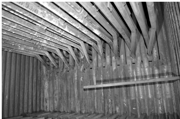
Figure 1: Part of superheater P1 and the membrane wall Slika 1: Del super grelca-pregrevalnika P1 in stena membrane
