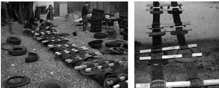
Figure 3: Tyrespace © project is another new structural games. In 2008, I led a Master workshop at the School of Architecture PUC in Santiago de Chile. In two weeks, 6 small groups produced a 12m span footpath bridge only with car tyres. They carried out several empirical tests using all the components and properties of each car tyre. The preliminary structural tests with strapping connectors failed. Those frames required extra-stiffness. Nevertheless the use of strapping methods showed capability to build up random tissue. Source: Dr. Suau archive (ECOFABRICA, 2012).
