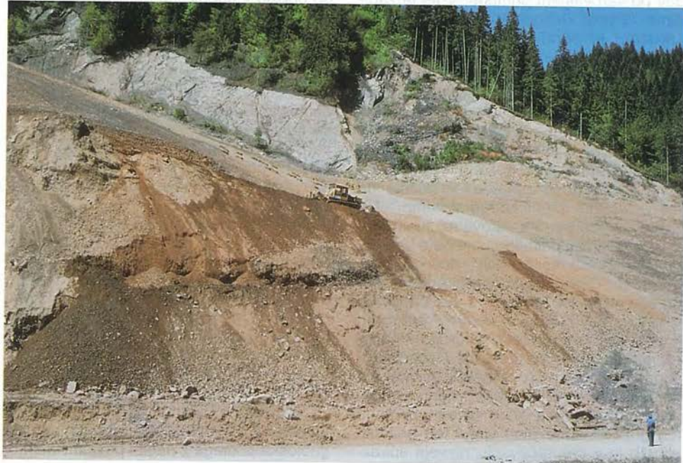
Dela na odkopavanju in izravnavanju površine plazne gmote (Foto A. Horvat) Excavation and levelling work on the area of landslide material (by A. Horvat)
