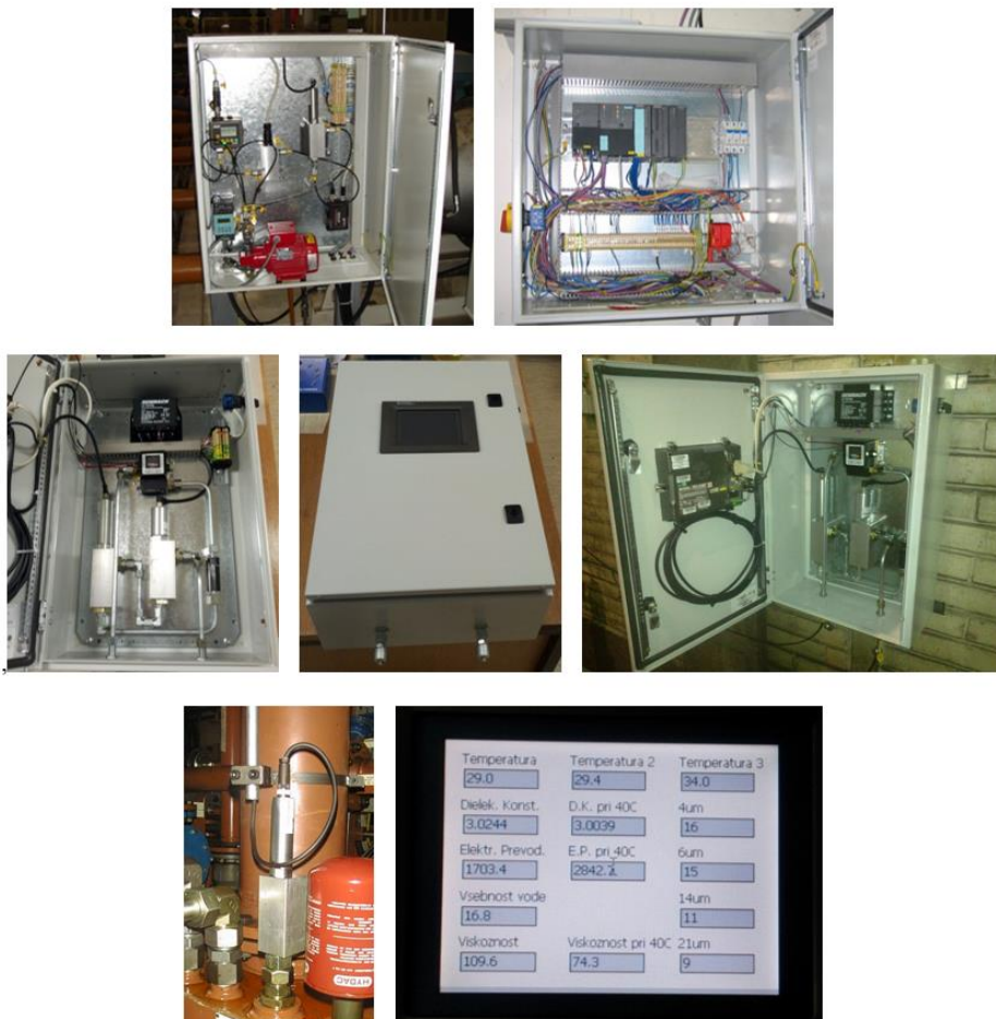
Figure 7.10: Different industrial applications of hydraulic oil condition monitoring, implemented during the studies in order to acquire real operating data
