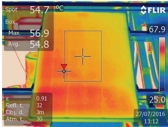
Figure 6: Thermo-vision pictures of the front side of the photovoltaic panel
