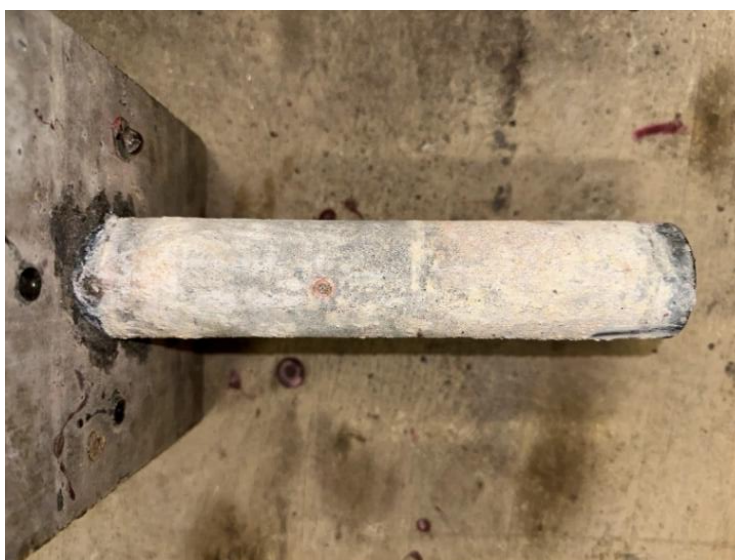
Figure 6: Expansive zinc-oxide development on the surface of a zinc-clad dowel.
