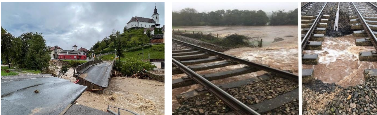
Figure 1: Photos showing extreme wash-out failures of roads and railway embankments: a collapsed bridge in Stahovica village, near the town of Kamnik, Slovenia (left) and flooded railway track in Herefordshire, Wales, UK (Network Rail, 2019) (right).
