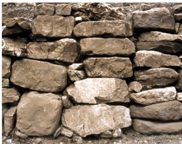
Sl. 153: Hiša 22. Gradbena faza 1, drenažni zid; pogled z juga. Fig. 153: House 22. Construction Phase 1, drainage wall; view from the south.
