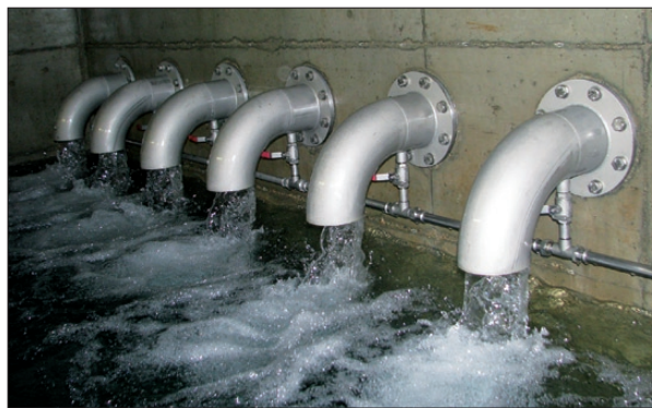
Fig. 2: Karst spring captured by means of inclined drillings and used for the drinking water supply of Yverdon-les-Bains, Switzerland. Providing safe drinking water at sufficient quality and quantity for all people is the major task and a permanent challenge for (karst) hydrogeologists (Photo: N. Goldscheider).
