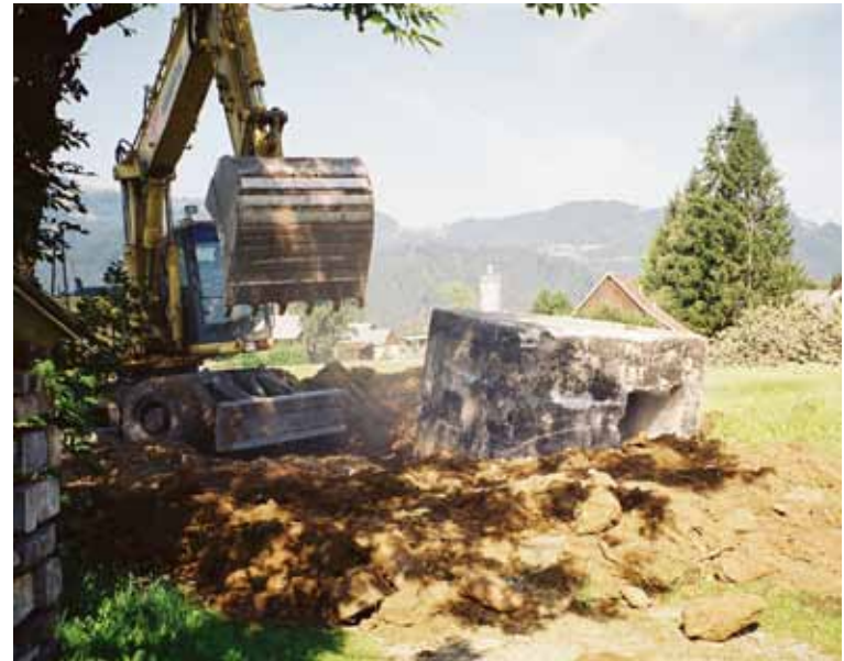
Figure 4: Until 18 September 2007 the bunker stood at the end of the street Pot na Koče. It was removed by Anica Likovič when the the road to the “Grugatova” house was built. It is now buried in the construction pit underneath the previous dirt road (author of the photograph: Zvone Kopač, 2007; source: author’s archives).
