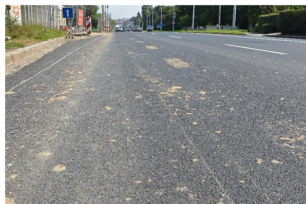
Figure 7: Clogging of road surface.
