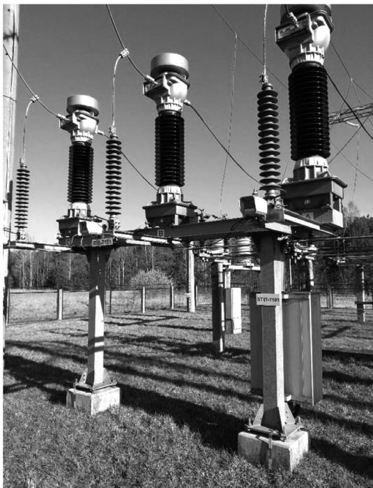
Figure 3: Object under investigation: a current and voltage transformer
