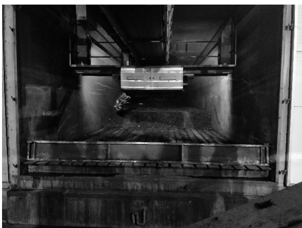
Figure 4: Compost tunnel with automatic filling system in operation
