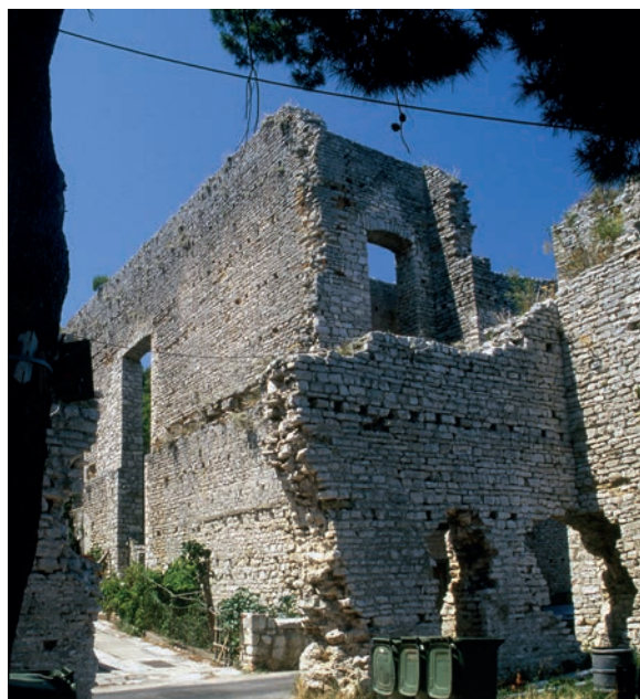
Fig. 3.43: Polače. Walls preserved to a great height from the eastern part of the villa (2005).
