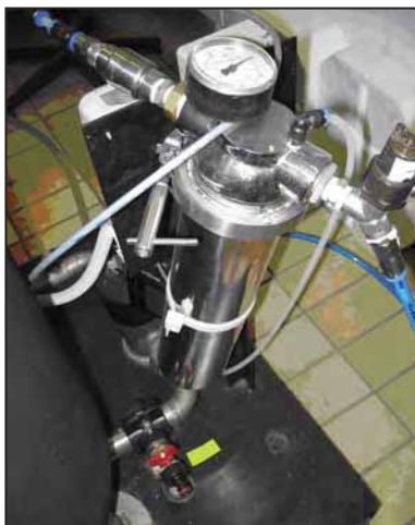
Figure 8. The additional gas reservoir.
