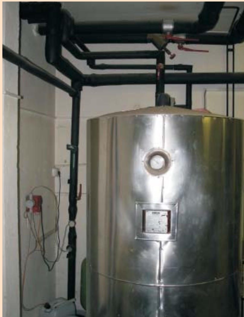
Figure 3: Sodium polyphosphates dosage into the drinking water system
