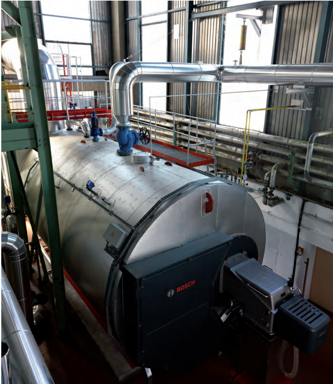
New steam boiler
