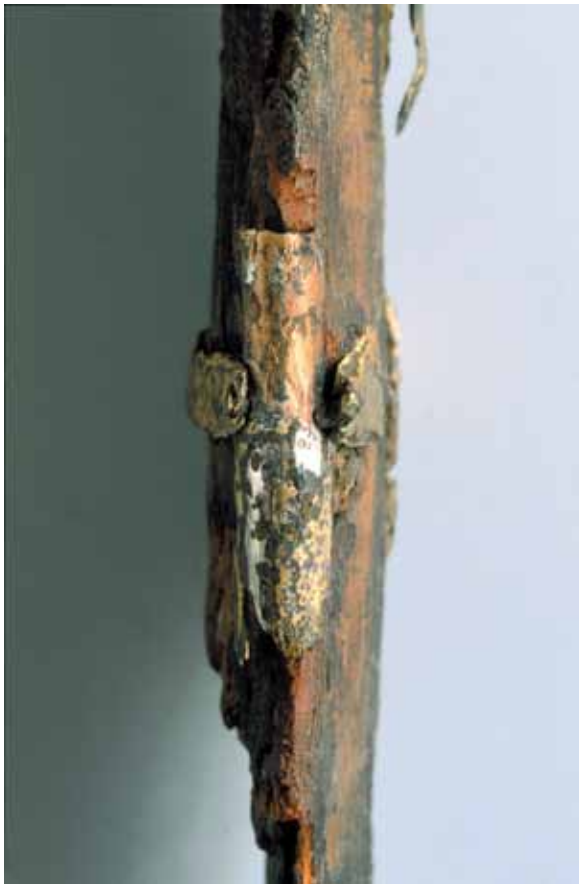
Fig. 5: The upper right solder-point of the guttering. Sl. 5: Spajkanje robnega okova na desni strani.
