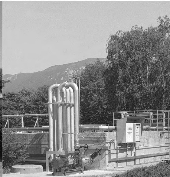
Fig. 7 Detail of one of the installed MIXFLO® system: pump, tubular oxygenator and control panels.
