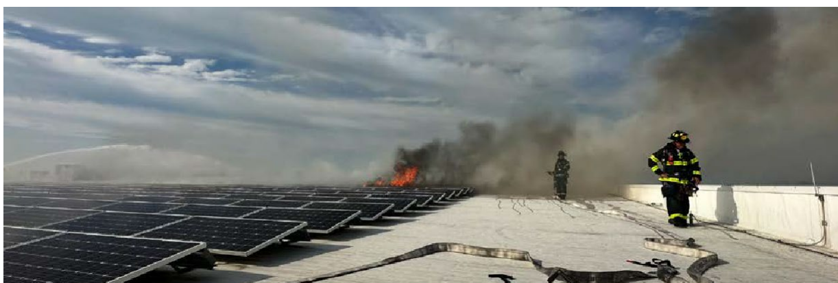
Vatrogasci gase požar na krovu s FN panelima u Robbinsvilleu (New Jersey, SAD) 2023.
