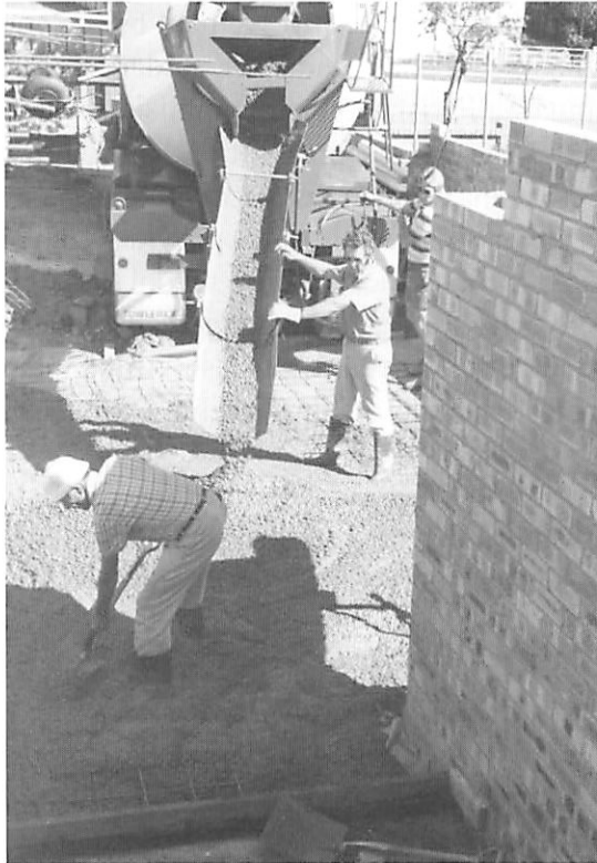
Work begins on the hall. Over a decade, the adjoining properties were purchased and the building of a hall was completed in 1983.
