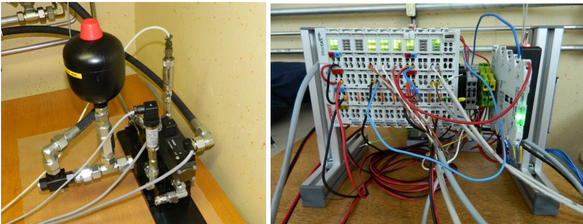
Figure 1: Physical construction of measuring track together with control device
