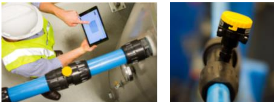
Figure 3: Advanced compressed air system condition monitoring - Transair® powered by SCOUT™ Technology
