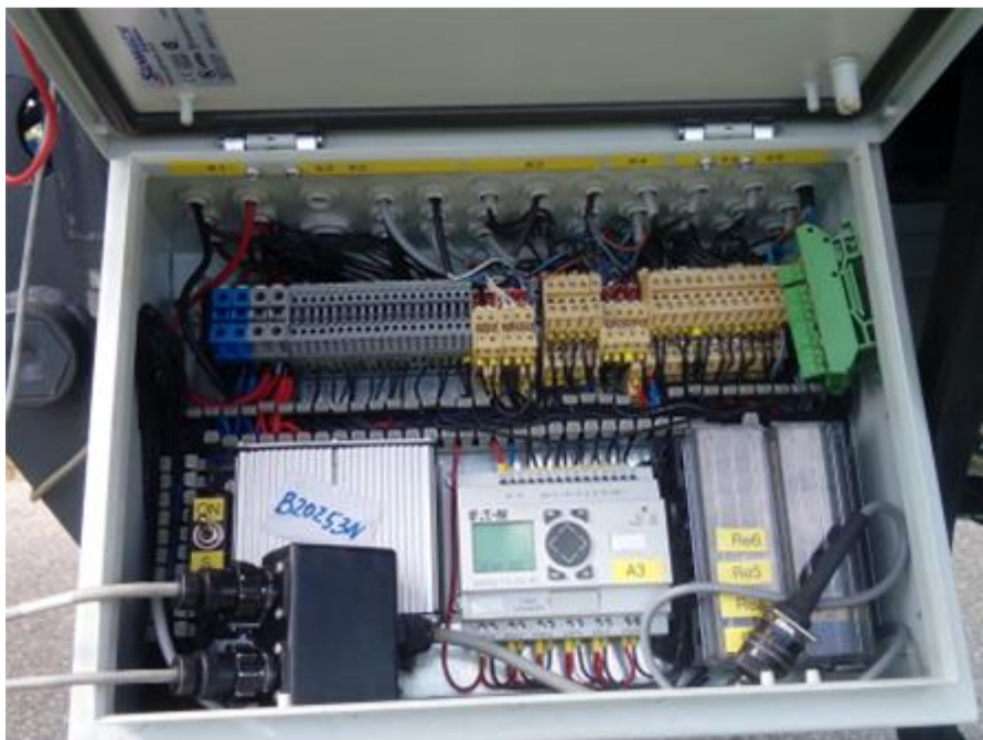
Figure 12: Trailer electro cabinet
