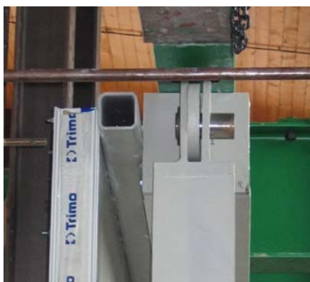
Slika 2.27: Detajl členkastega vozlišča ter pritrditve lege in panela Figure 2.27: Detail of the pinned hinge and fastening of the rafter and panel
