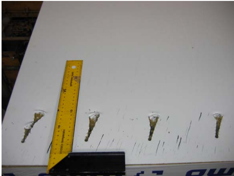
Slika B.23: Pretrg notranje pločevine zunanjega panela Figure B.23: The tear of the inner steel sheeting of the outer sandwich panel
