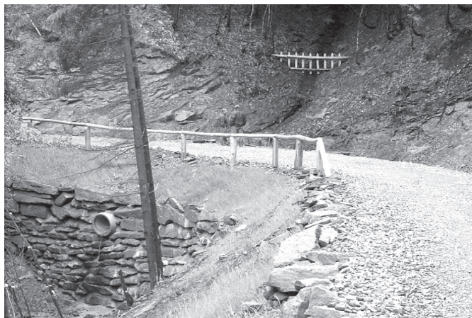
Slika 8: Primer kakovostne graditve gozdne ceste Figure 8: An example of well constructed forest road
