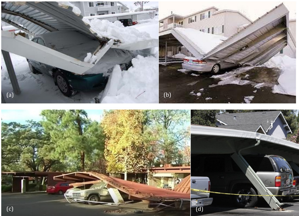
Fig. 3 Structural failure of carport structures due to snow load – (a) and (b), wind load (c), earthquake (d) [16-19]
