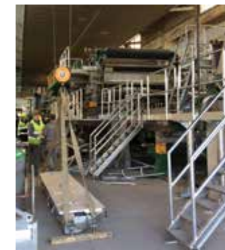
Prenovljeni mokri del KS2 med prenovo Renovated wet end of the KS2 cardboard machine during renovation
