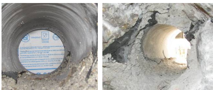
Slika 5.39: Vrtina in globinska sonda izvedena v spodnji polovici zidu 4-C2 Fig. 5.39: Borehole and in-depth probing at the lower half of the wall 4-C2
