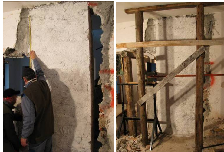
Slika 5.23: Izmera zidu 3-AC2 in izvedene lesene podpore Fig. 5.23: Measurements of the wall 3-AC2 and executed wooden supports
