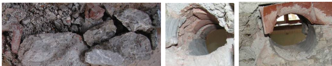
Slika 5.36: Jedro in globinske sonde, izvedene na zidu 3-AC2 Fig. 5.36: Core and in-depth probing at the wall 3-AC2
