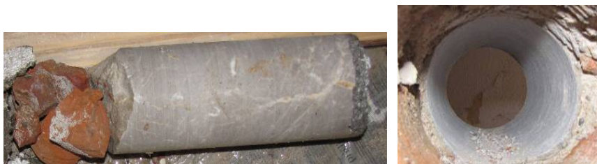
Slika 5.33: Jedro in vrtina, izvedena v zgornjem delu zidu 2-AC1 Fig. 5.33: Core and in-depth probing at the upper part of the wall 2-AC1
