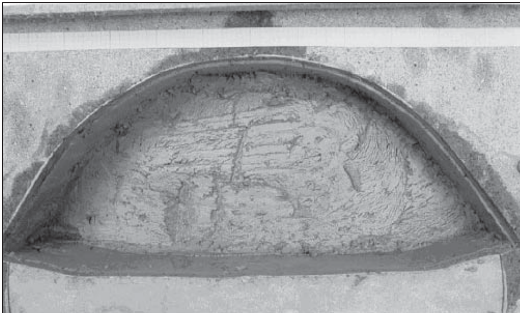
Figure 3. Appearance of deformation.
