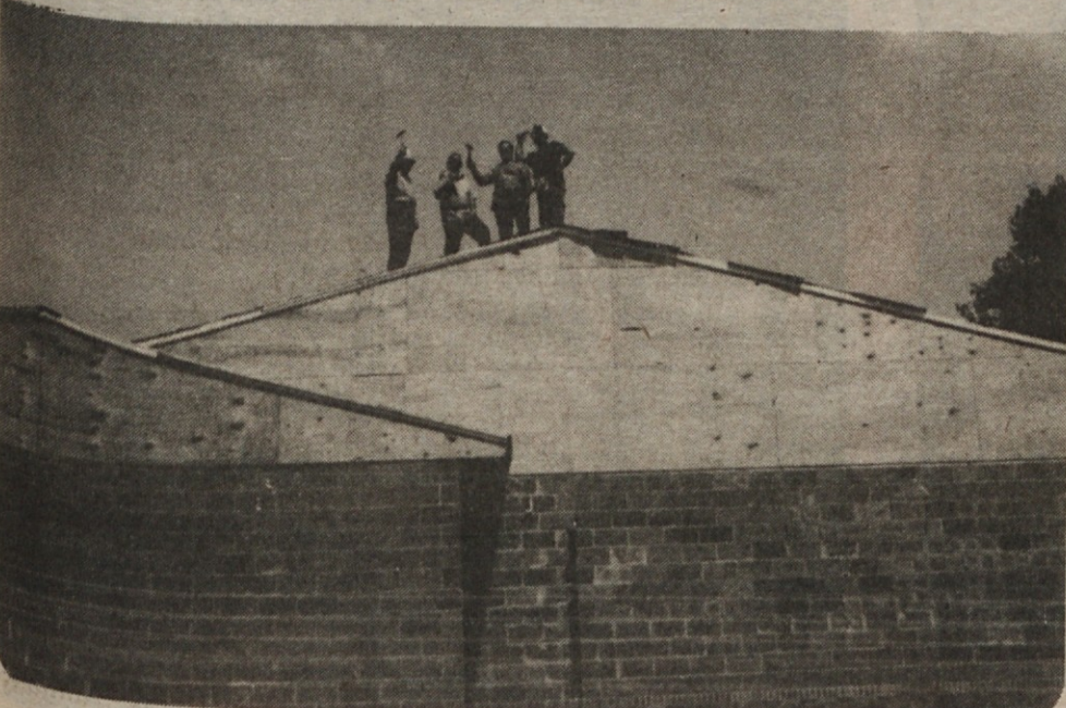
Taking a view from our new roof top as the roof sheathing is being installed,
