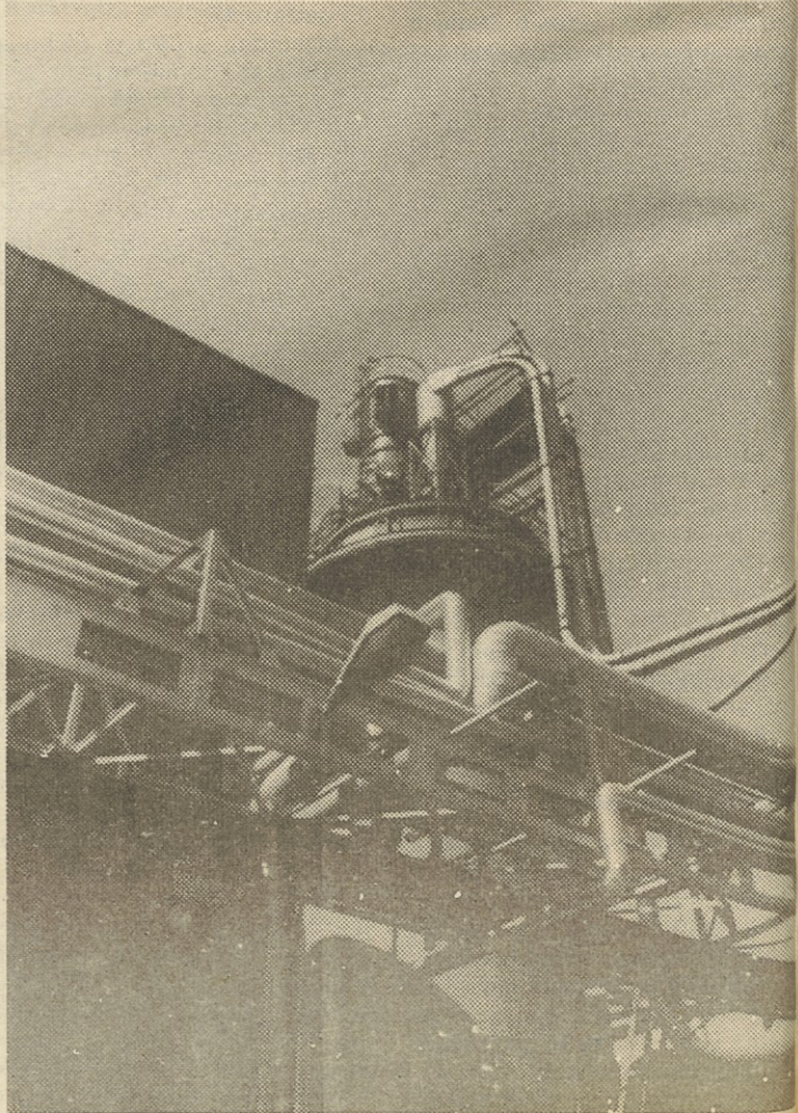
Filter montiran nad silosom
