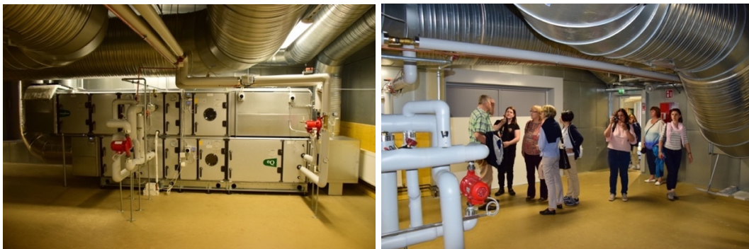
Figure 5: MEP room (source: InAirQ team)
