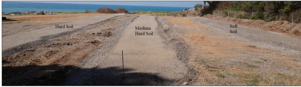
Figure 1. Preparation of soft, medium hard and hard soil pits for post installation.
