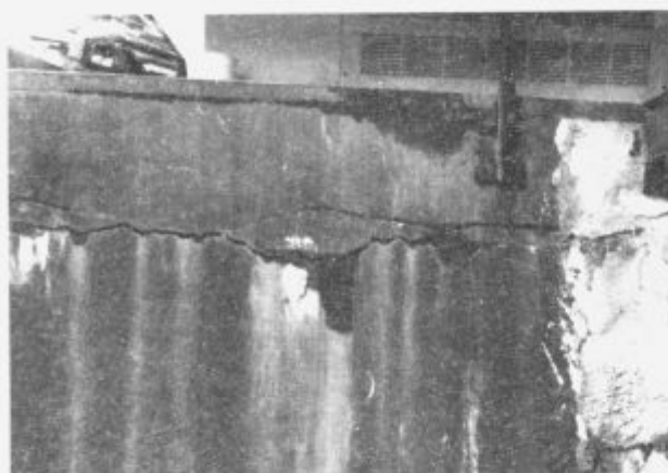
Slika 2: Detajl na poškodovanem objektu Figure 2: Detail on damaged construction
