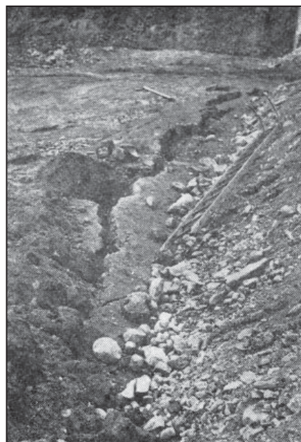
Figure 1. Longitudinal crack on the surface of the clay core – Jirkov dam.
