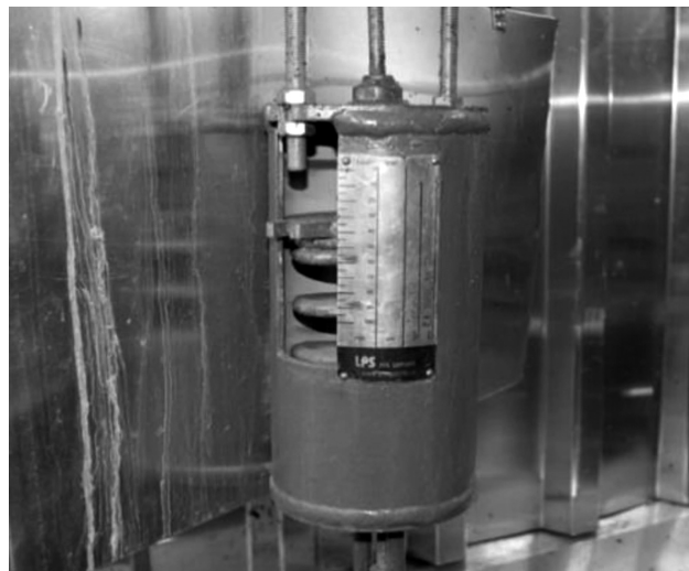
Figure 3: Spring support of the transition pipe Slika 3: Vzmet v pretočni cevi
