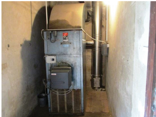
Figure 3: Boiler room with ELFO boiler
