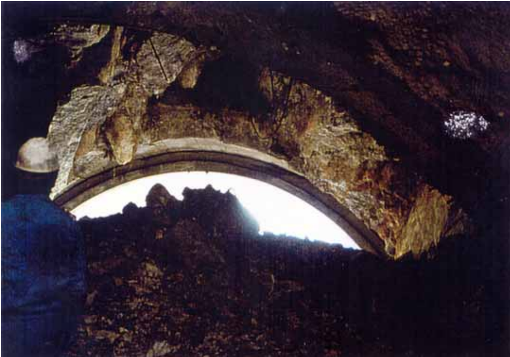
Figure 5. Slide of a dolomite block in the Golo rebro Tunnel at chainage 27+974 [2] Slika 5. Zdrs dolomitnega bloka v predoru Golo rebro na stacionaži 27+974 [2]
